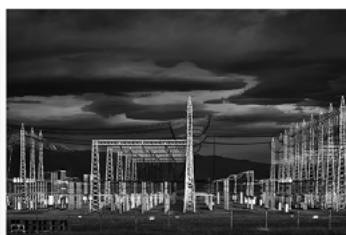
Twizel Sub Station Late light flatters off the substation's highly reflective towers, contrasting against a dark and brooding sky to the west.
